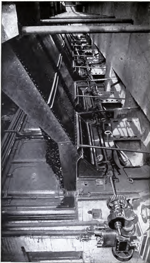
Roney Mechanical Stoker, Showing Coal Delivery Shuttles and Operating Engine.
